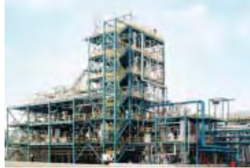
Photo 2 One-hundred ton/day demonstration plant
